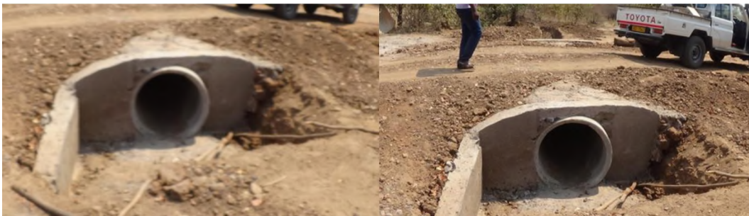
Figure 7.2: One of the culverts constructed in Chadereka by community members. Source: Rosemary Kasimba
