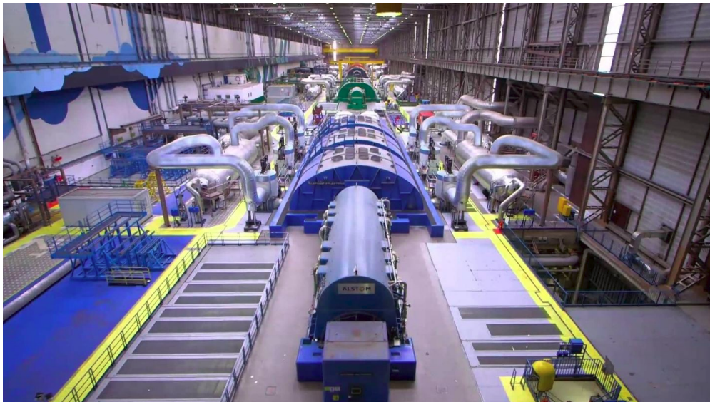
Figure 5.3.: A turbo generator in the engine room of a nuclear power plant
