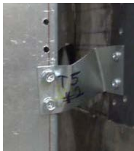
(a) Later-torsional buckling
