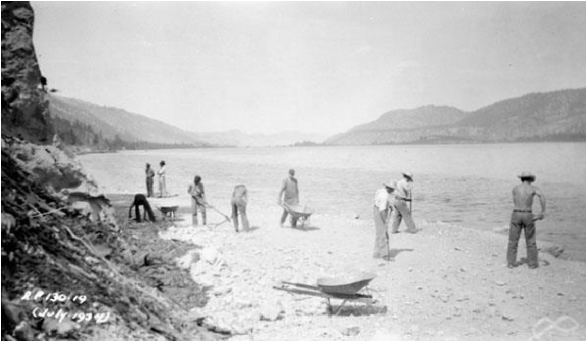
Figure 2.5: This image of a highway work crew highlights the difficult terrain in the Okanagan. (Photographer unknown. “(Relief Projects – No. 130). Widening the Kelowna-Vernon Highway.” Image No. PA-037242. Photo courtesy of the Canada Department of National Defence / Library and Archives Canada. Copyright expired.)
