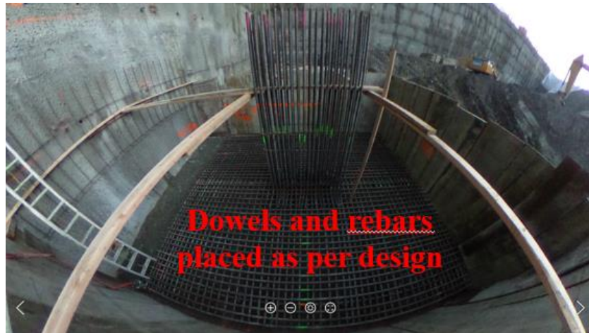
Figure 6.14: Sample image highlighting how small structural elements are reviewed remotely using only spherical images.
