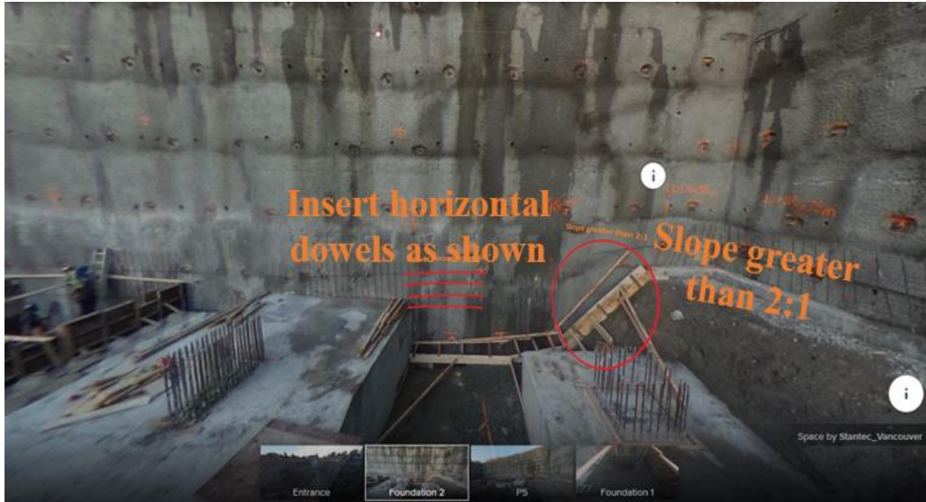
Figure 6.12: Sample image highlighting how the structural design related issues are reviewed and communicated with team members using only spherical images.
