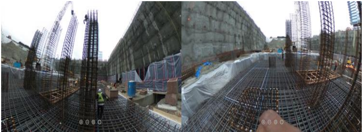
Figure 6.13: Sample images highlighting the significant amounts of rebar in the shear wall foundation that needs to be reviewed occasionally.
