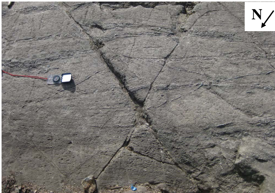
Figure 29. Conjugate fracture set on a horizontal wall. The compass is 17 cm long.
