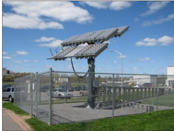
Figure 2-15: The SUNRISE demonstrator at NREL, Ottawa Canada. [15].
