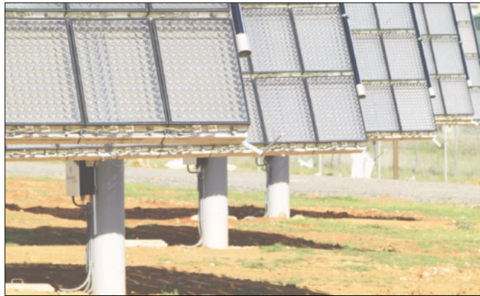
Figure 2-19: Concentrix solar array.[46].
