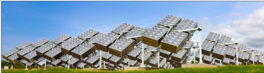
Figure 2-17: An array of Emcore CPV systems with tilt and roll tracking and silicone on glass lens [46].
