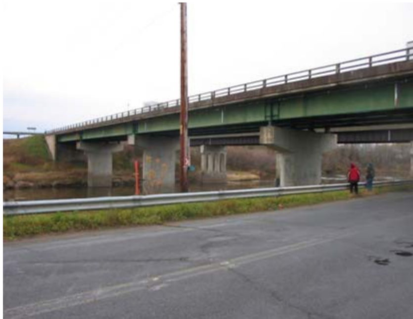
Figure 4.8: Madrid Bridge (Guizani, 2007)
