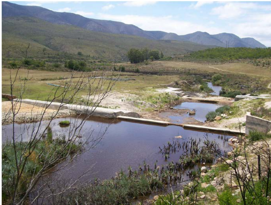
Figure 3.9: Cement weirs built along the Kromme River, Eastern Cape, South Africa. These weirs are built to restore the river by stopping the headcut from proceeding backwards up the river. This traps sediments and allows vegetation, such as P. serratum in this photograph, and eventually wetlands to recover
