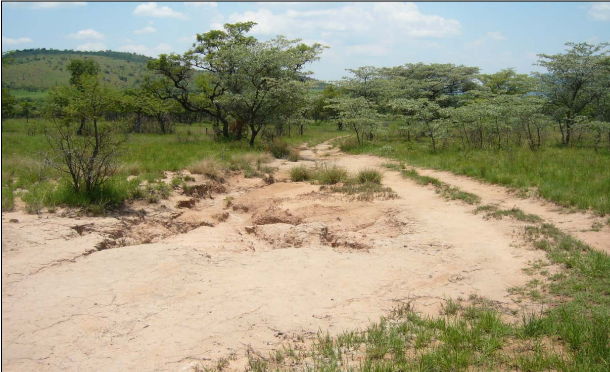
Figure 7.3 Poorly planned and constructed roads lead to erosion
