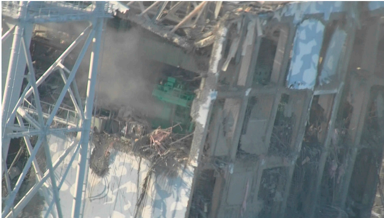
FIGURE S2.1 Photograph of Unit 4 obtained during the March 16, 2011, helicopter overflight of the Fukushima Daiichi site. The photo shows the refueling deck region in the vicinity of the spent fuel pool. The green equipment visible in the center of the image is the fuel handling machine. SOURCE: http://photo.tepco.co.jp/en/date/2011/201103-e/110317-01e.html .
