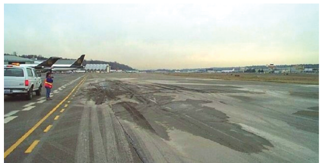
FIGURE 4 Nisqually Earthquake, February 2001, sand boils, Boeing Field Taxiway, Seattle, Washington. (Photo credit: M. Anderson.)
