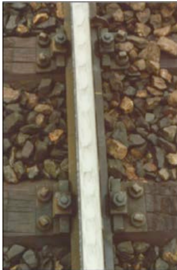
FIGURE 5 Short wave formation (corrugation control). (Source: INNOTRACK final report.)
