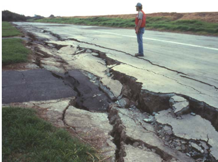
Figure 5: Roadway damaged from lateral spreading in 1989 Loma Prieta earthquake (from Nakata et al., 1990)
