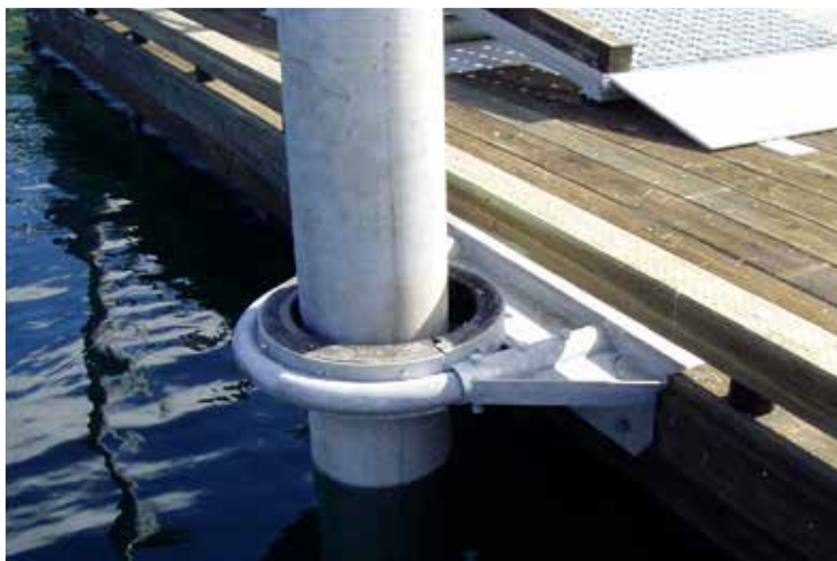
FIGURE 18 Example of a galvanized steel floating dock attachment. (Credit: V. Skagerberg, Alaska DOT&PF. Used with permission.)
