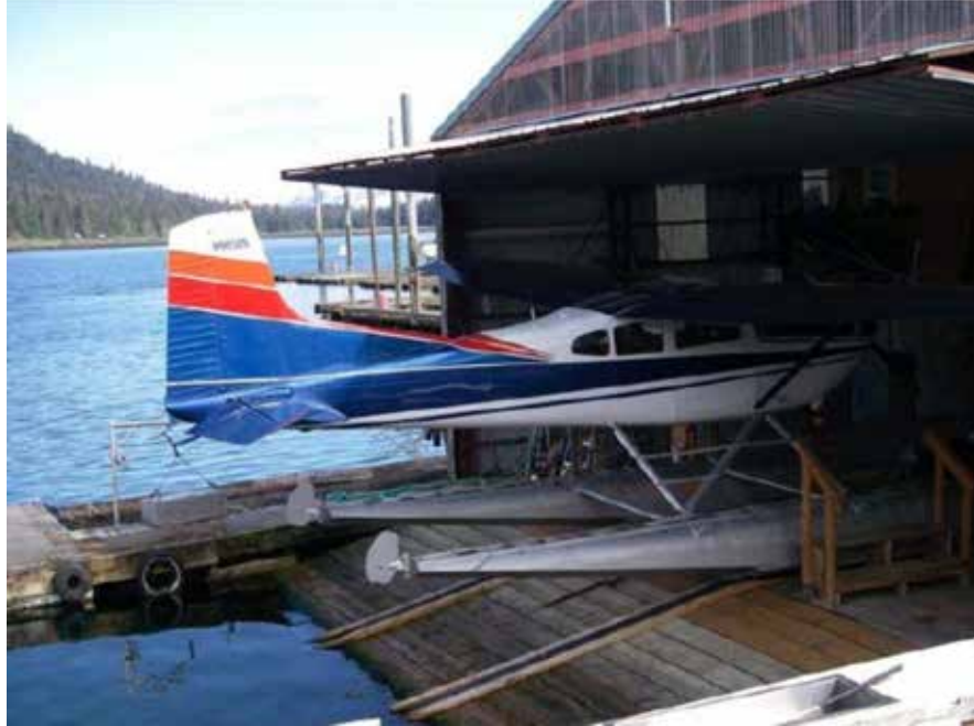
FIGURE 13 Floating hangar with ramp and rail dolly system. [Source: Alaska DOT&PF (Siting Analysis, Sitka Seaplane Base—Sitka, Alaska 2012)]
