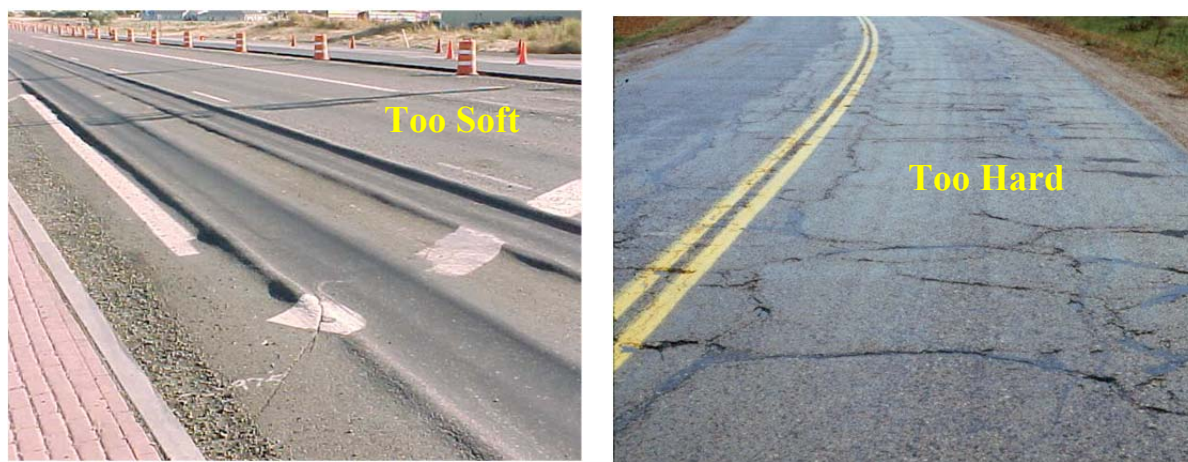
FIGURE 1 Examples of issues with too hard or too soft mixes.
