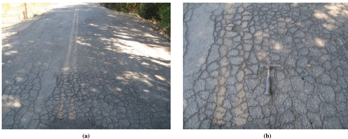
FIGURE 1 A failing asphalt road (a), and a close-up showing breakup of the pavement surface (b). (Photos courtesy of D. Jones.)
