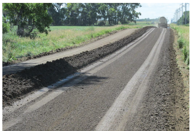
FIGURE 5 Active conversion of a failing pavement by adding new gravel and recycling. (Photo courtesy of K. Skorseth.)
