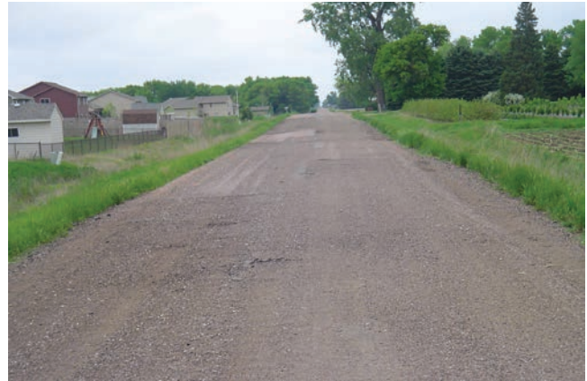
FIGURE 7 A township road failing because it carries heavy loads for which it was not designed. (Photo courtesy of K. Skorseth.)
