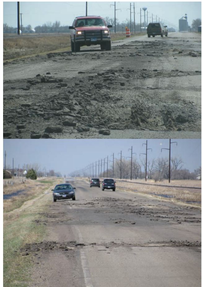
FIGURE 8 Examples of road safety effects caused by failing asphalt roads. The failures force traffic to travel outside of the lane and disrupt traffic movement. (Photos courtesy of K. Skorseth.)
