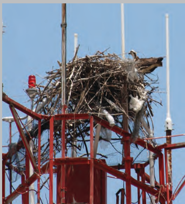
Osprey nesting on a communications tower at a southeastern U.S. airport.
