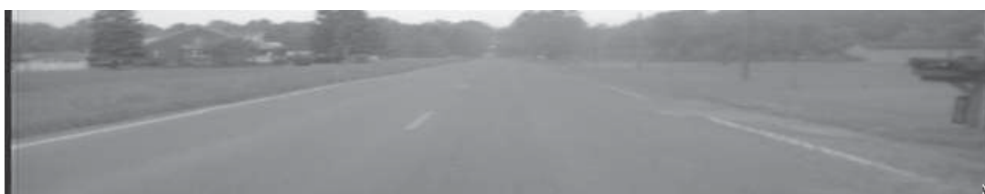
Right pavement markings indicated as “obscured.”
