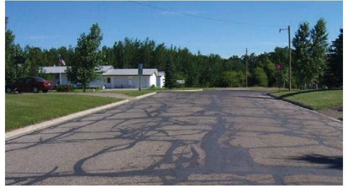
Photograph 2-2. Excessive crack filling (photo by Dale Decker).
