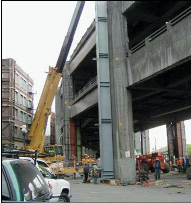
Figure 32. WSDOT crews repairing earthquake damage on the viaduct in April 2001 (Credit: WSDOT).
