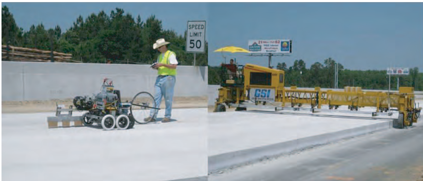
Figure 2.18. Hardened concrete measurements with Ames Engineering RTP (left) and GOMACO GSI (right).
