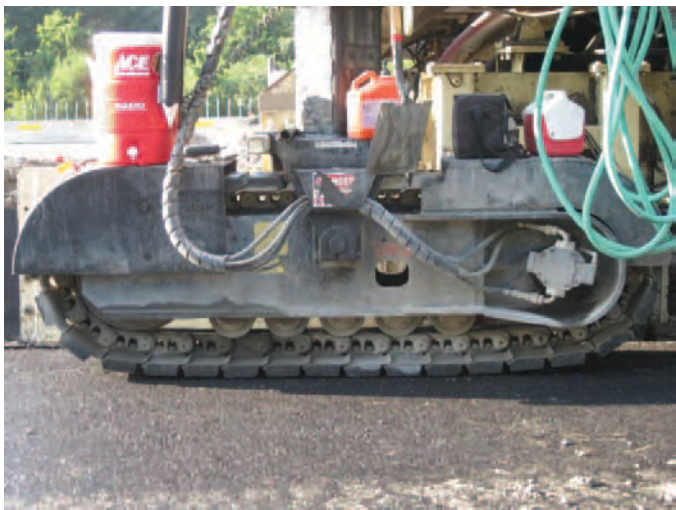
Figure 2.67. Length of paver track is a possible explanation of a repeating feature in New York profiles.
