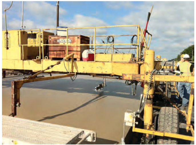
Figure 2.65. Additional RTP equipment supplied by Ames Engineering mounted to a work bridge.
