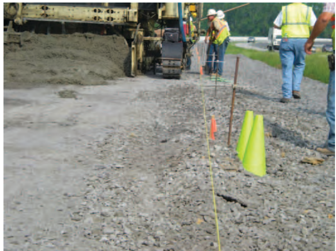
Figure 2.42. Paver track line deviation resulting from unstable subgrade conditions.
