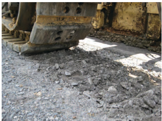
Figure 2.43. Soft material in paver track line at location of localized roughness.
