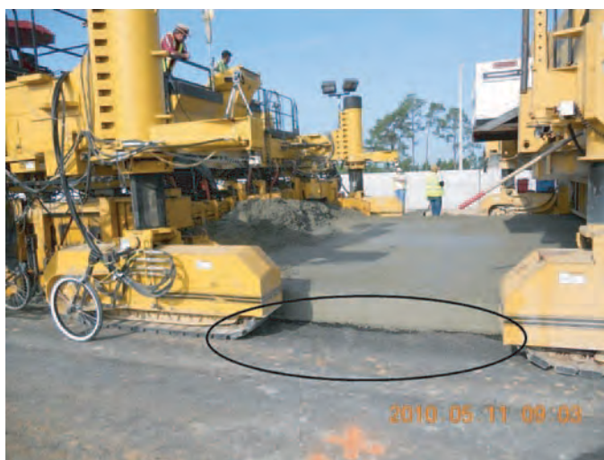
Figure 2.27. Bump in the right track line at Station 509+00.
