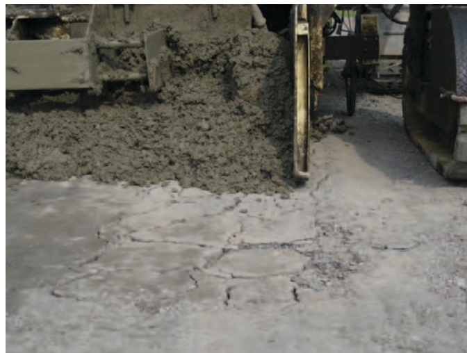
Figure 2.45. Failure in HMA interlayer at location of localized roughness.
