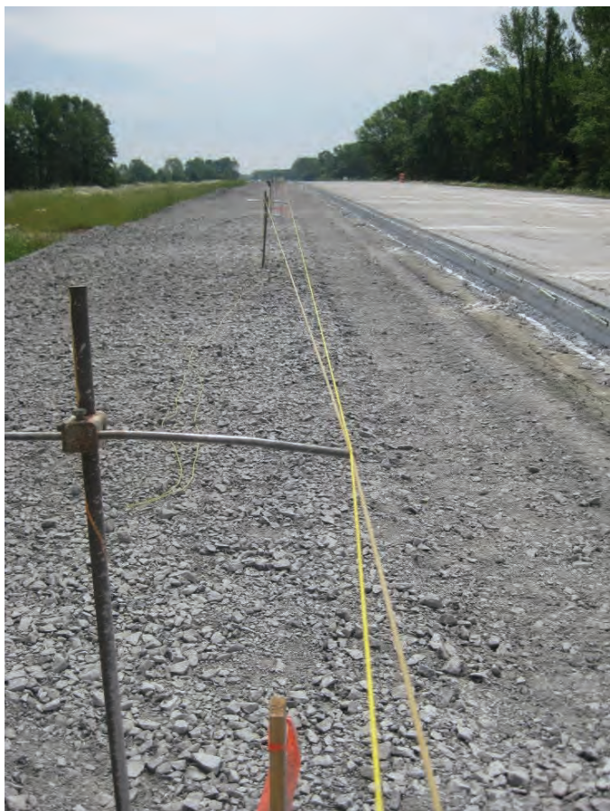
Figure 2.44. String line splice at location of localized roughness.
