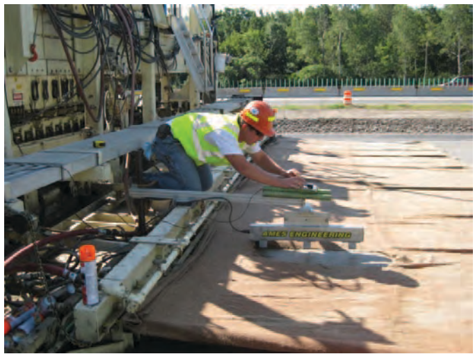
Figure 2.69. Location of Inertia-Link sensor with respect to the paver-mounted Ames Engineering RTP, with dowels used for mass dampening.
