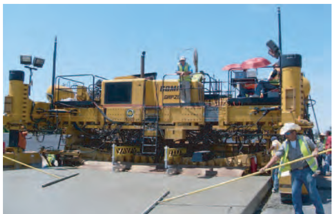
Figure A.6. Rear view of GOMACO GHP 2800 slipform paver and hand finishing.
