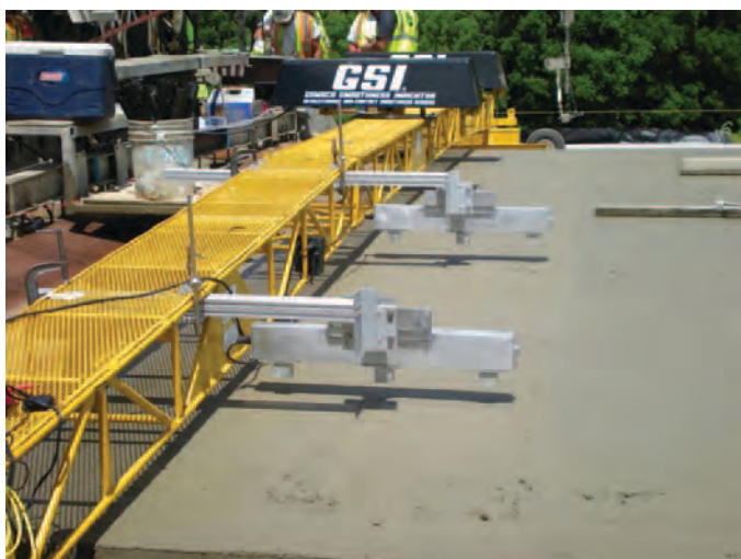
Figure 2.52. GOMACO GSI and Ames Engineering RTP mounted to a work bridge towed by the paver.
