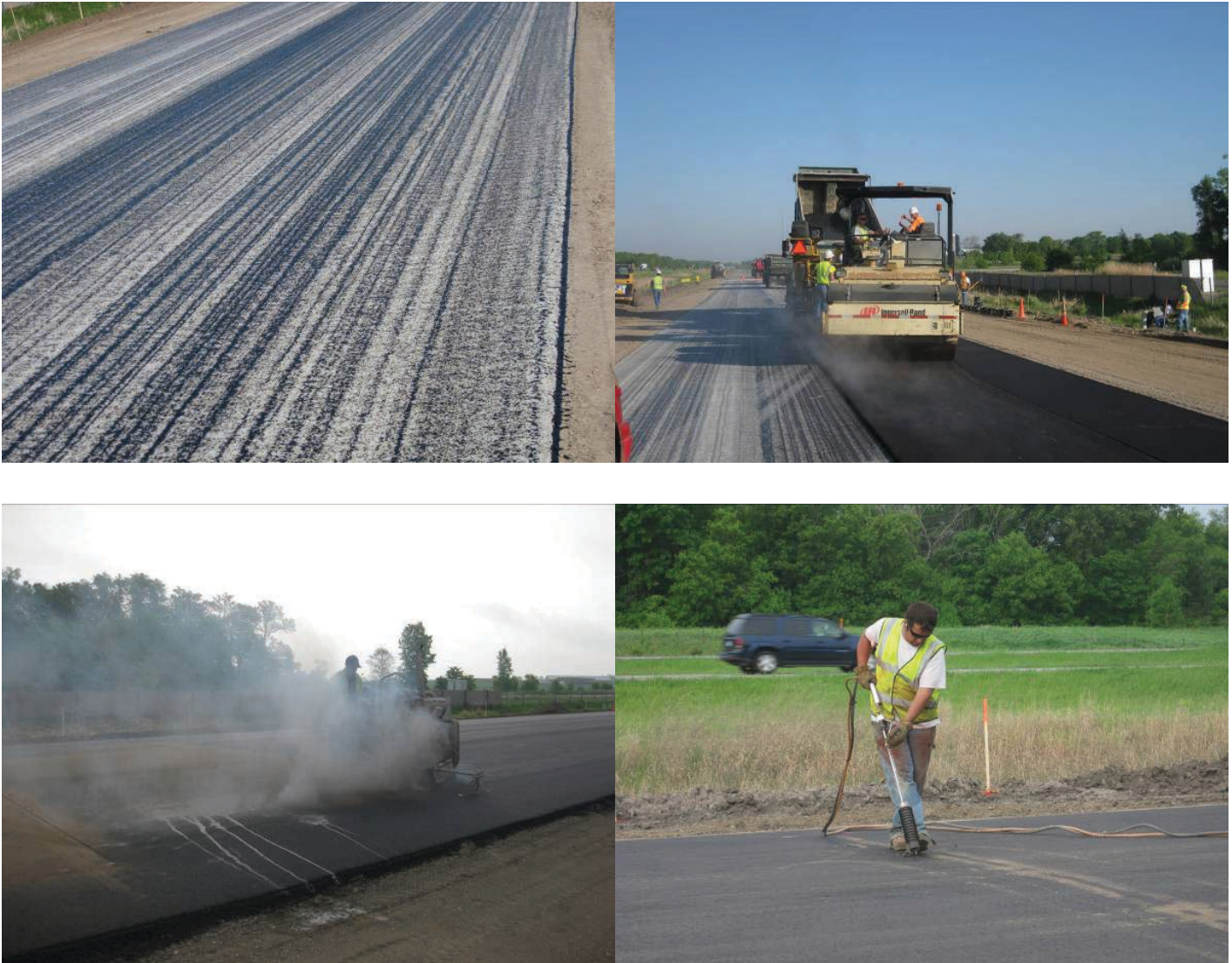
Figure 2.20. Tack coat applied to PCC surface (top left) prior to HMA paving (top right). Sowing (bottom left) and sealing (bottom right) HMA layer; saw cuts in the HMA were matched to the saw cuts in the PCC below to within 12.5 mm (0.5 in.).
