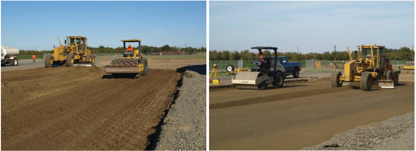
Figure 5.1. Grading and compacting the subgrade and base in preparation for PCC placement.
