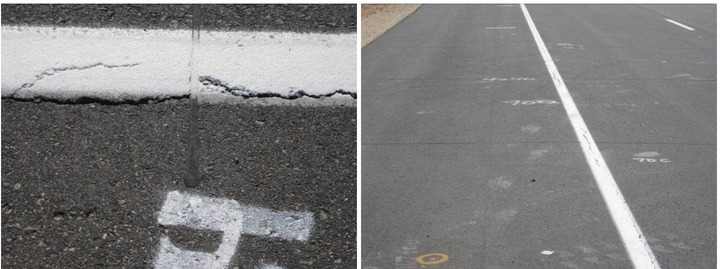
Figure 5.8. Saw cut and sealing of the HMA surface can be extended partially or completely into the HMA shoulder.
