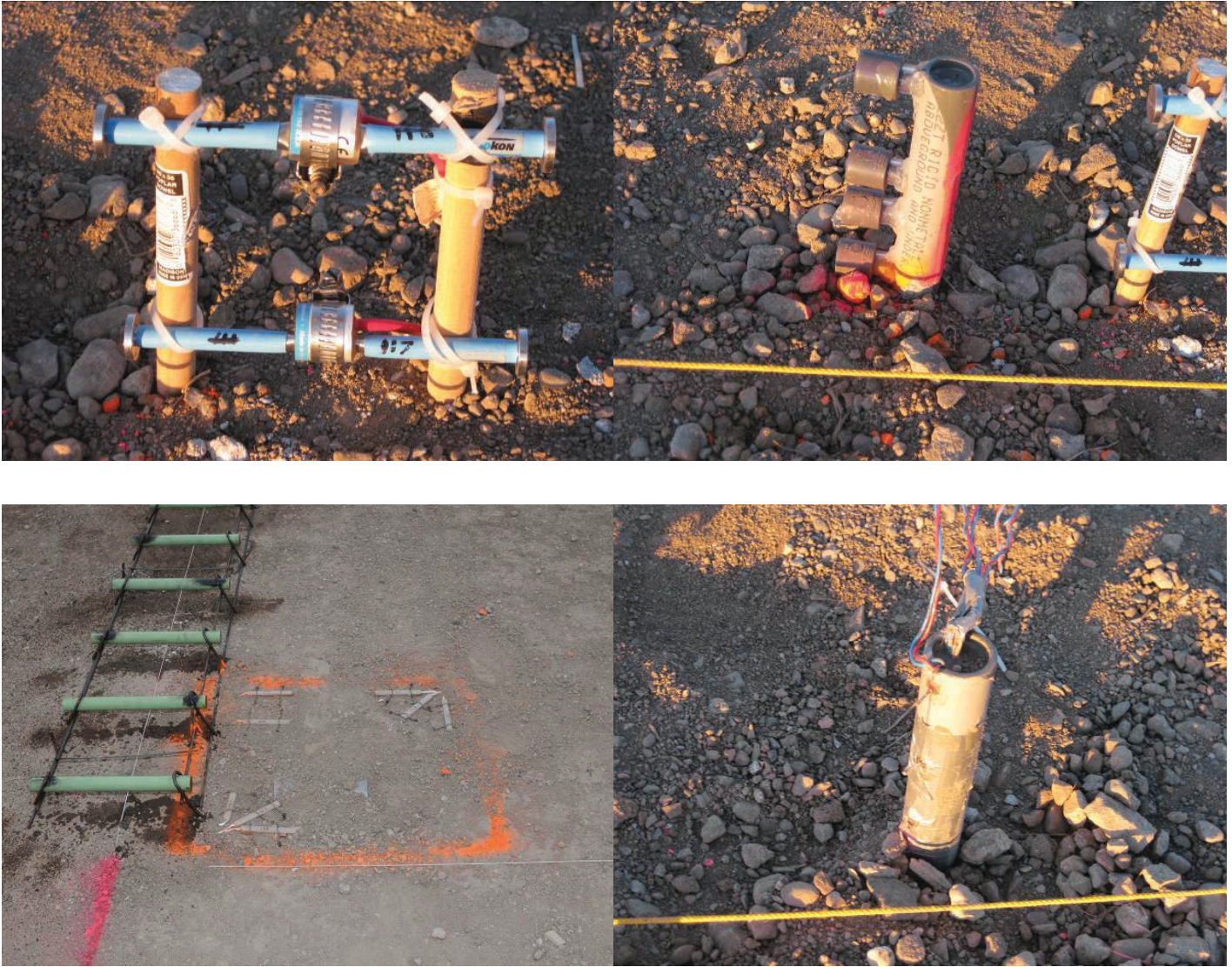
Figure 2.14. Instrumentation installed prior to placement of the PCC to measure pavement responses to temperature and traffic loads (static strain gauge, top left; dynamic strain gauges, bottom left; humidity sensors, top right; temperature sensors (thermocouple tree), bottom right).
