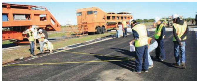
Figure 2.35. Measurement of the positions of strain gauges on first lift of PG64-28PM, before placement of second lift.
