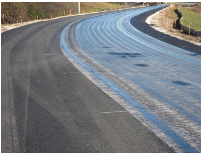
Figure 2.40. Application of tack coat on PCC and marking the shoulder (to identify saw cut locations for sawing and sealing HMA).
