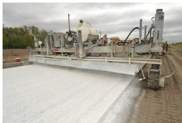
Figure 2.19. Applying curing compound to the surface of the PCC to control surface drying of the PCC and minimize early age distresses.
