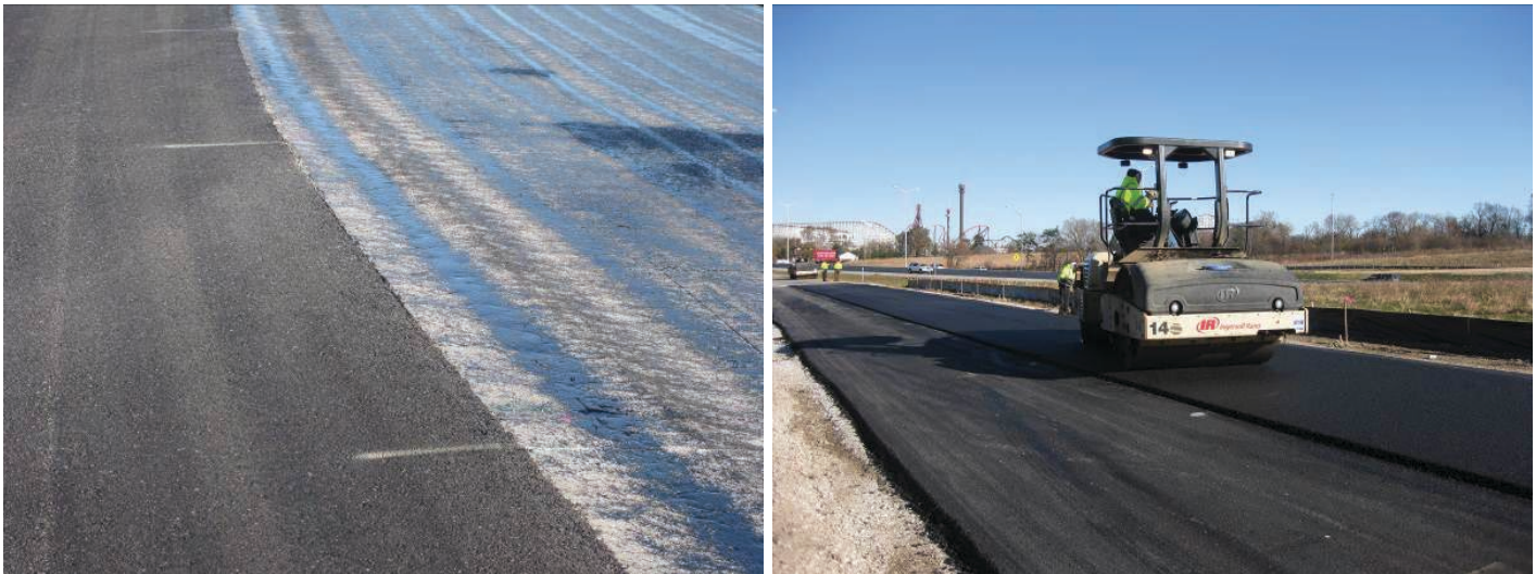
Figure 5.5. This figure demonstrates marking location of sawed joints in PCC at a location that will not be covered by the HMA so the HMA can be sawed and sealed at the same location.
