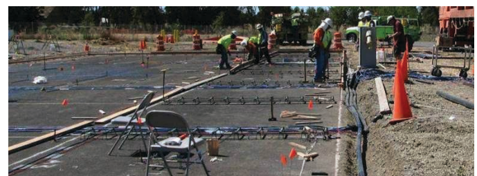
Figure 2.27. Track overview showing sensor wires fixed to track.
