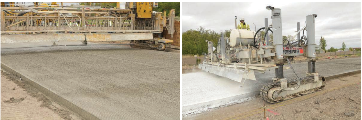
Figure 5.4. Longitudinal tining texture and curing compound applied to the wet PCC surface to ensure mechanical bond between the HMA layer and the PCC layer and control surface moisture loss.
