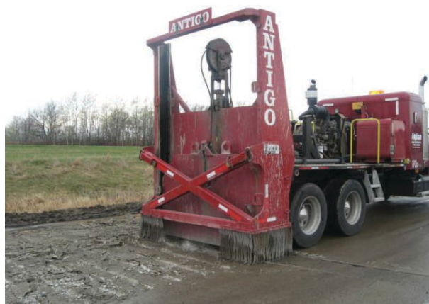
Figure 2.5. Guillotine crusher breaking existing concrete for recycling into the PCC layer of the HMA/PCC composite pavement.
