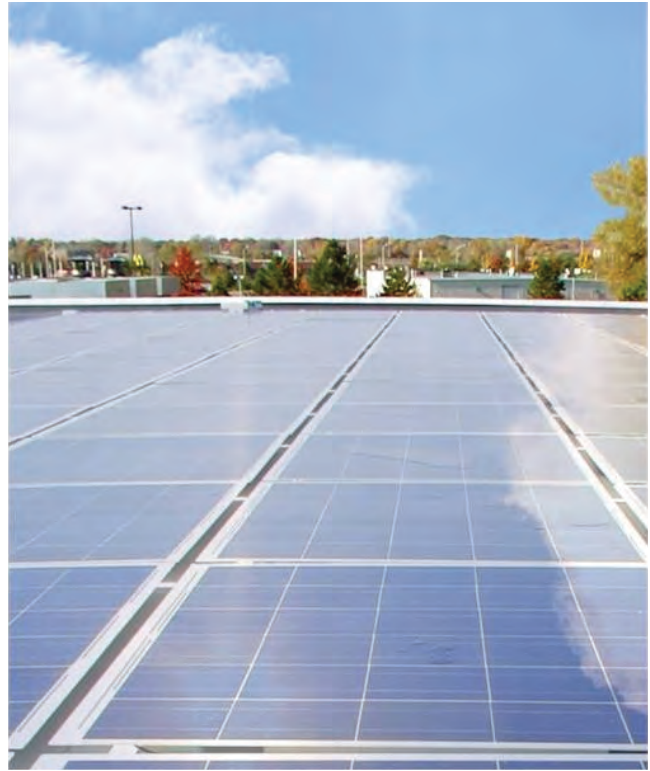
FIGURE 13 CT Transit's solar array.
