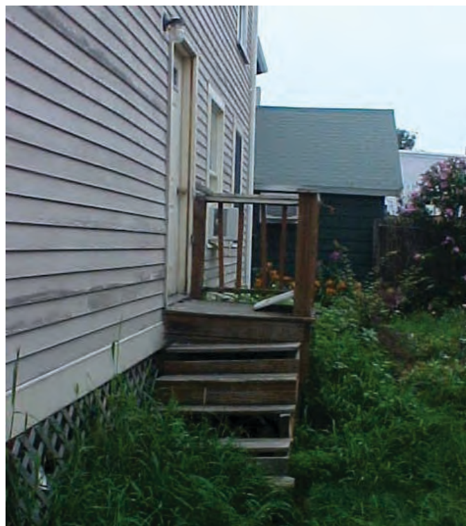
Figure 5.15. Door landing in poor condition.
