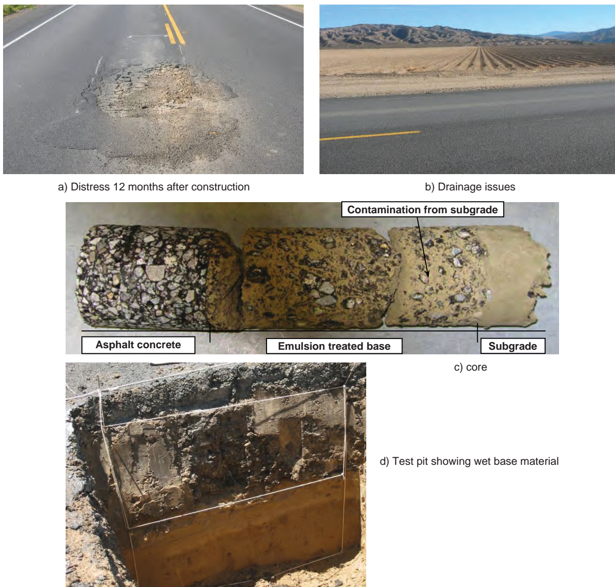
Figure B.3. Investigation photographs for Case Study 3.
