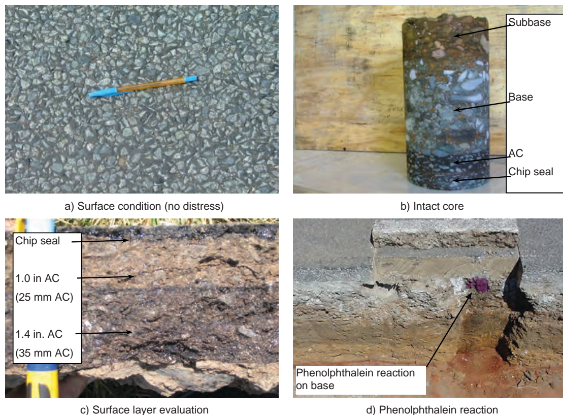
Figure B.1. Investigation photographs for Case Study 1.
