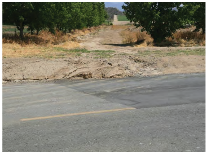
Figure 4.6. Access road drainage problems (note digout).
