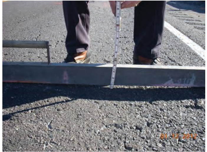
Rutting in the problem area
