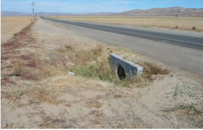
Figure 4.2. Blocked side drain and culvert.
