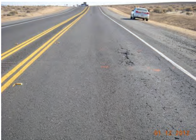
View of distressed area
