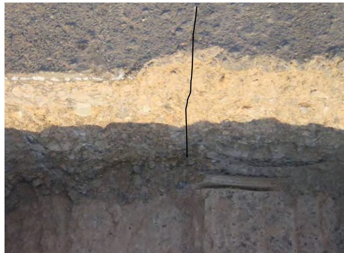
b) Vertical crack to mid point in reclaimed base
