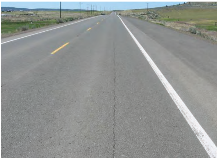
a) Longitudinal crack on surface
