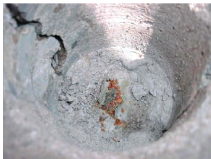
Dowel bar failure/corrosion seen in core hole
