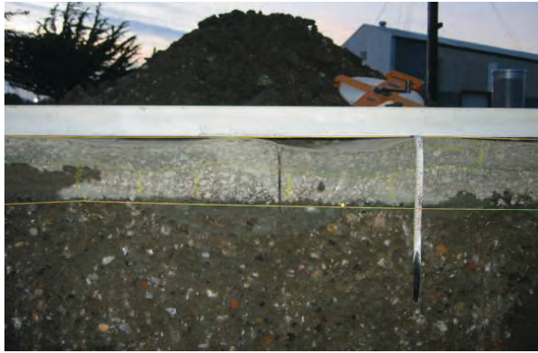
a) Note rutting in underlying AC layer.
