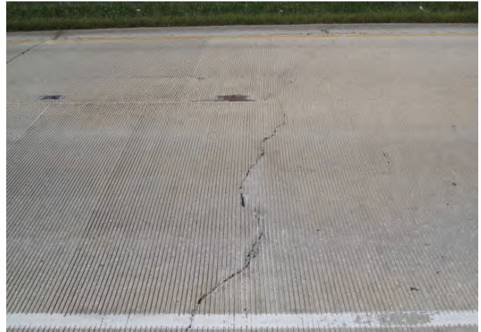
b) Mid-slab crack
