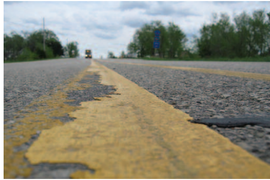
Close-up view of yellow line deterioration.
