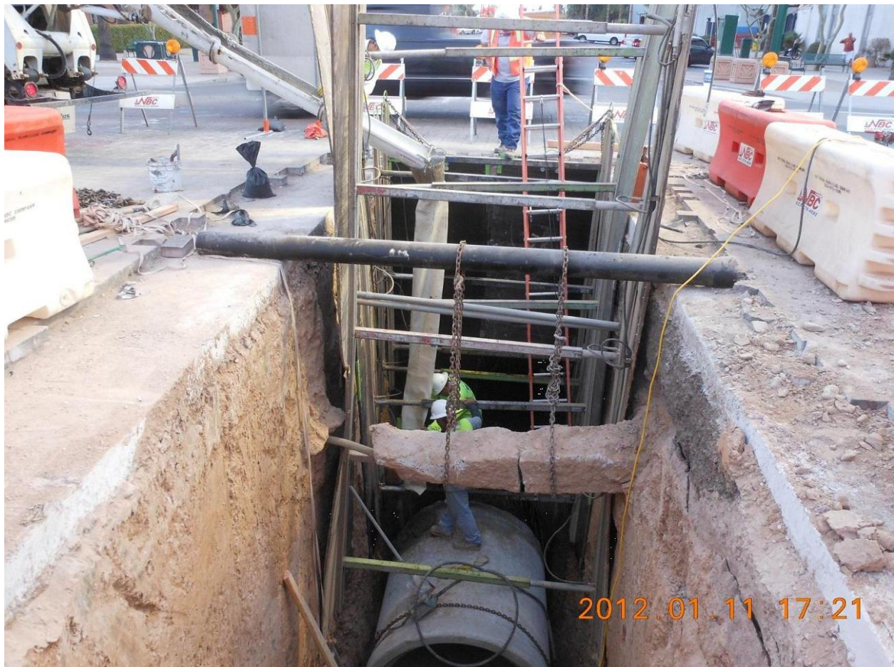
FIGURE 1 Here is a simple example of installing offset manholes to maintain access to an existing 84-in. storm main left in place below a light rail. A main thrust of SUE is integrating qualified data with design and construction to engineer protect-in-place strategies for existing utilities. The SUE process promotes damage prevention, cost and schedule reduction, commerce interests, and above all, the public welfare.
