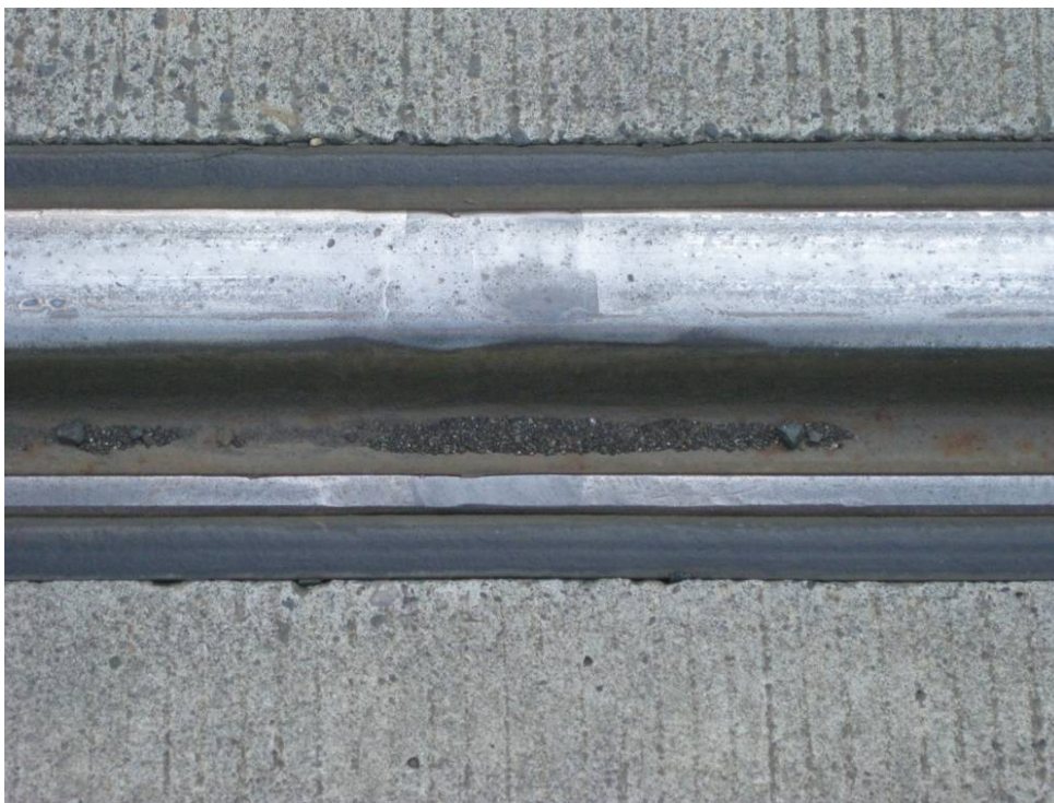
FIGURE 12 Rail condition in Portland (12).
