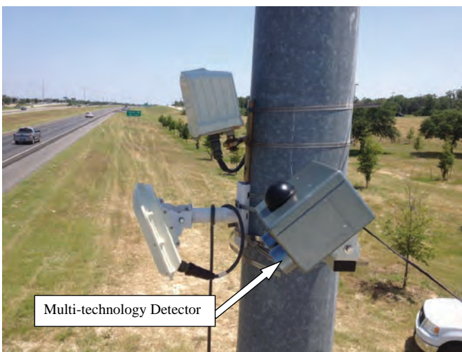
Figure 4. Multi-technology detector mounted at SH 6.
