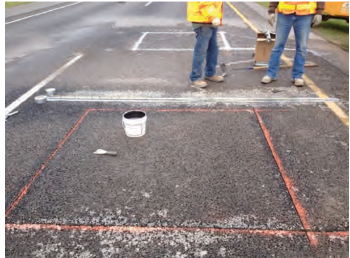
Figure 2. Inductive loops and piezoelectric sensors installed in SH 6.
