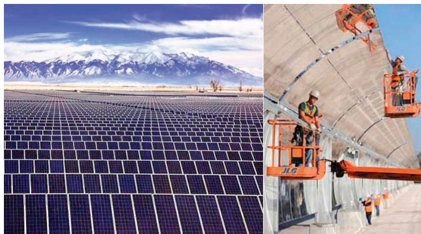
FIGURE 3.1 (Left) Utility-scale PV system . (Right) Construction of concentrating collectors for the Martin Solar Plant (a concentrating solar power system). SOURCE: (Left) http://solarpanelspower.net/solar-power/the-politics-of-solar-power . (Right) Sherwood (2011).
