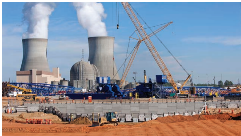
FIGURE 2.13 New construction at an existing two-unit nuclear power plant. SOURCE: © Southern Company, http://www.southerncompany.com/nuclearenergy/photos.aspx .
