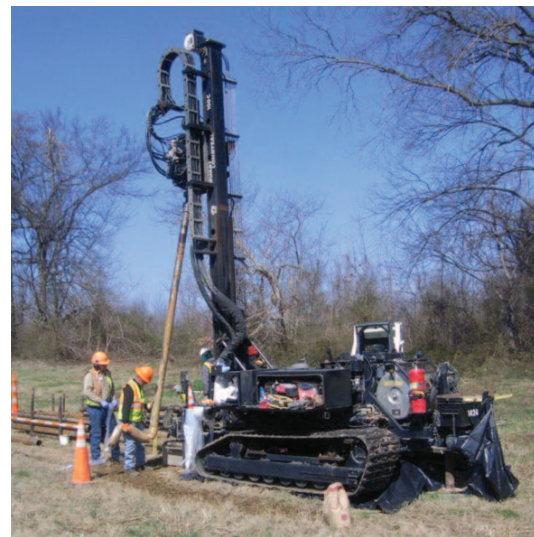
Track-mounted rotosonic drill rig operating south of the landfill. The crew is extruding a sample from a 95-ft geotechnical boring into a flexible plastic sleeve.
