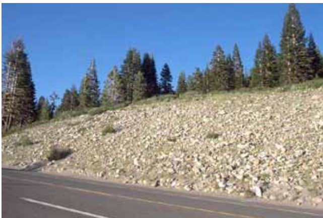
FIGURE 18 Rock blanket on a cut slope for erosion control, Lake Tahoe (Courtesy: G. Keller).
