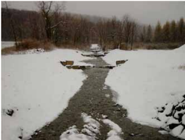
FIGURE 20 Stone check dams (Courtesy: D. Orr).
