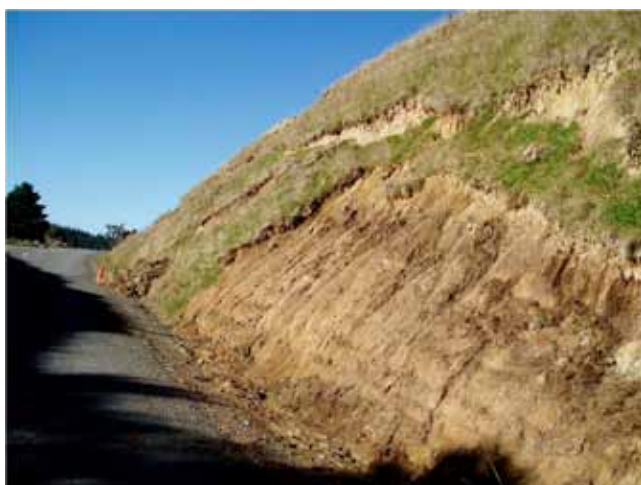
FIGURE 4 Shallow cut failure just below grass root depth. Use deep-rooted vegetation for slope stabilization (Courtesy: G. Keller).
