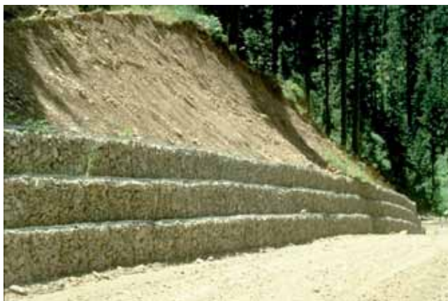
FIGURE 35 Low gabion wall and gabion wall stabilization at top of fill slope in Timor (Courtesy: G. Keller and C. Bennett).
