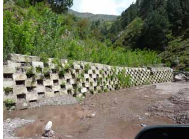
FIGURE 29 Post-earthquake (2005) slope stabilization using a masonry crib wall and layered planting of native trees and bushes, Balakot-Kaghan Road (N-15), Pakistan (Courtesy: A. Faiz).
