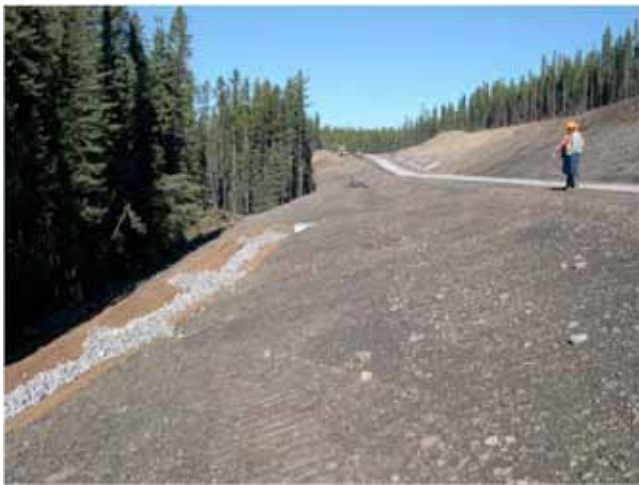
FIGURE 9 Geotextile- and rock-lined ditch example of surface drainage (Courtesy: C. Gillies).
