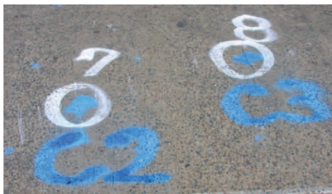
Figure 5.12. Vertical crack and core locations.
