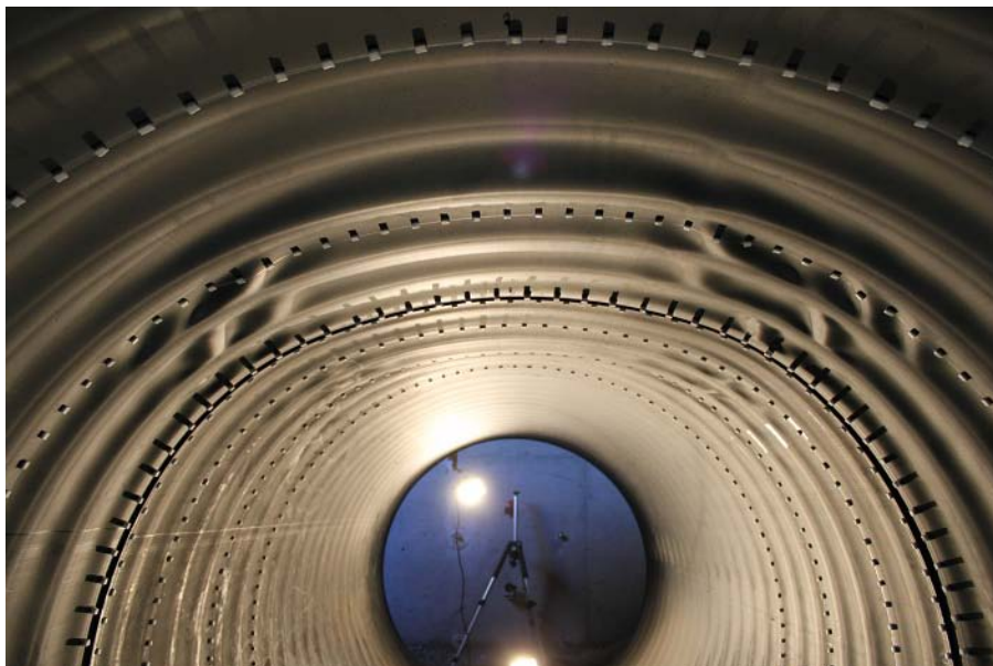
Figure C.97. HDPE pipe after ultimate limit state test.
