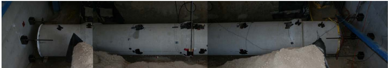
b. Photograph of experiment showing end plates anchored to the walls of the test pit
