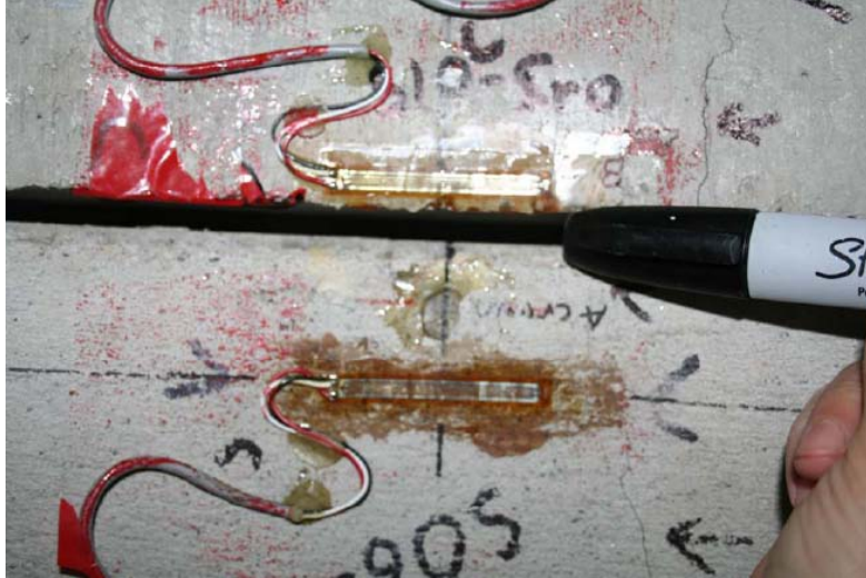
Figure C.27. Close-up of the crown of the 24 in. (610mm) diameter reinforced concrete pipe at the central joint; joint open about 0.5 in (12.5mm).
