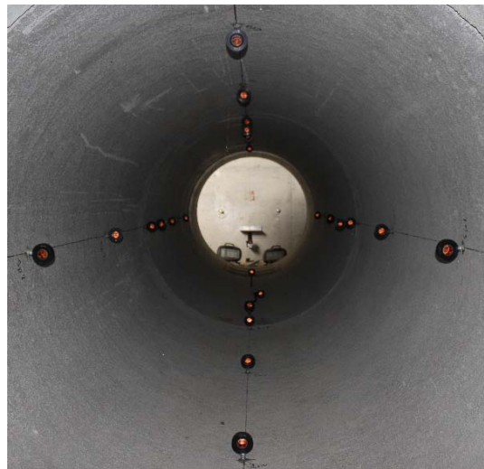
Figure C.11. View of the prisms after placement in the 48 in (1220mm) diameter reinforced concrete pipe.
