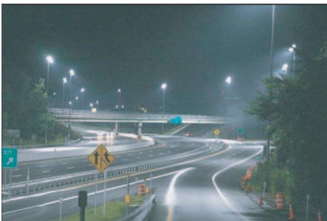
Figure 3.12. Test stretch for high-mast lighting (Freyssinier et al. 2008, photo Dennis Guyon, Lighting Research Center).
