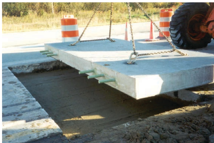
Figure 2.3. Variation of intermittent repair technique with slots for dowel bars cut in existing concrete pavement.
