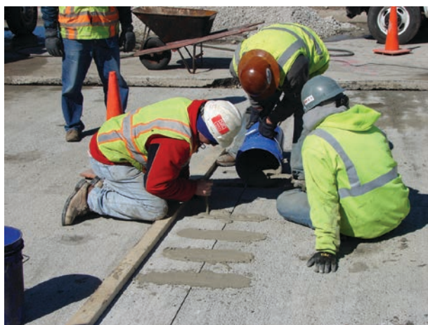
Figure 2.4. Variation of intermittent repair technique with dowel bars installed after panel installation using DBR method.
