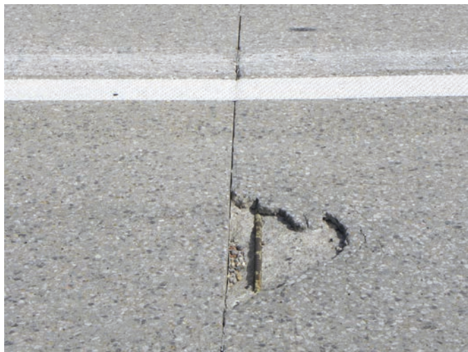
Figure 3.19. Spalling at an intermediate transverse joint on I-57 in Missouri.
