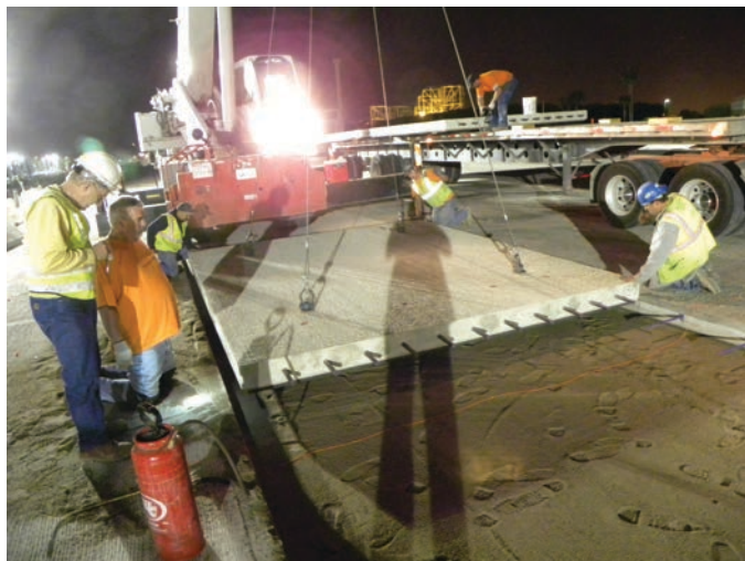
Figure 6.3. Footprints indicate a poorly compacted fine-grained bedding layer.
