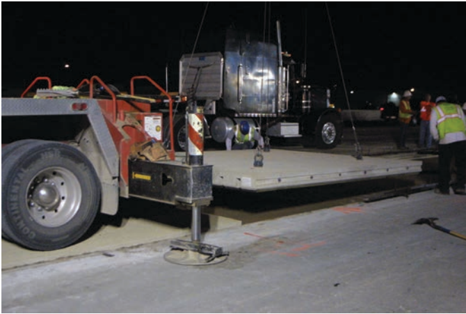
Figure 15.6. Crane stabilization requires 2 to 3 additional feet away from the rehabilitation lane on each side.
