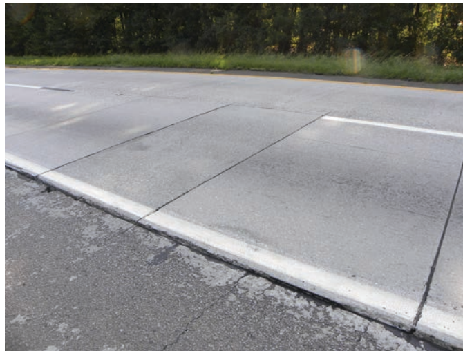
Figure 14.4. View of I-95 jointed FDRs in South Carolina.
