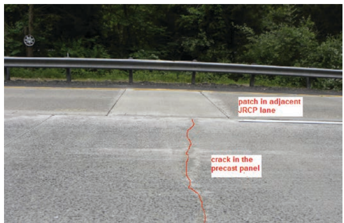
Figure 3.11. Crack in a precast panel associated with a patch in the adjacent lane on I-66 in Virginia.
