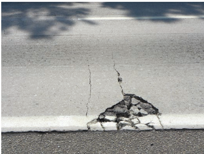
Figure 14.1. CRCP punchout distress.
