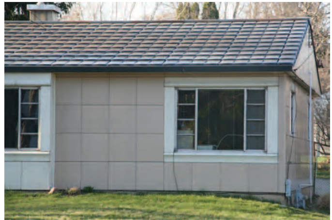
Figure 95. Porcelain enamel coated steel panels on a c.1950 Madison, Wisconsin, Lustron home (Mead & Hunt photograph).
