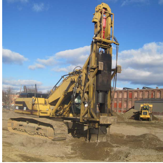
Rapid impact compactor in the process of compaction. From the files of P. Becker.
