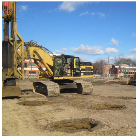
Rapid impact compactor following first pass of compaction points. From the files of P. Becker.
