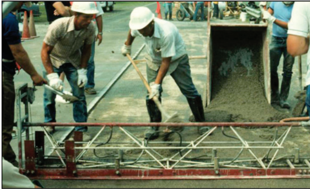
FIGURE 6 Vibrating screed consolidates and strikes off PPC overlay. (Courtesy: Virginia Center for Transportation Innovation and Research.)
