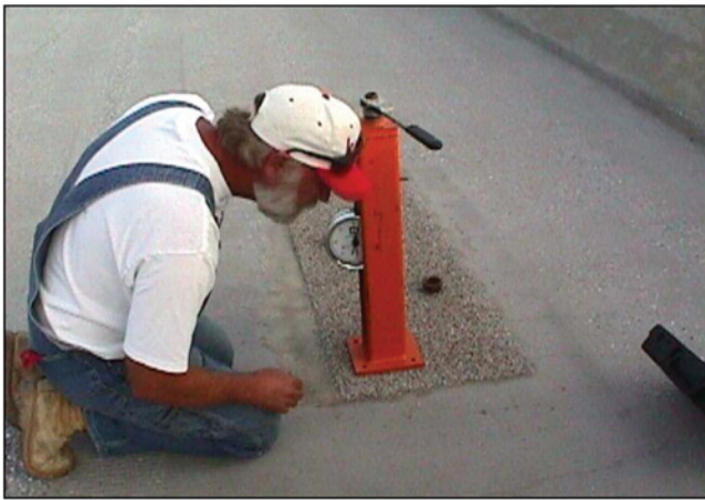
FIGURE 16 Pull-off test to determine suitability of surface preparation or bond strength of overlay.
