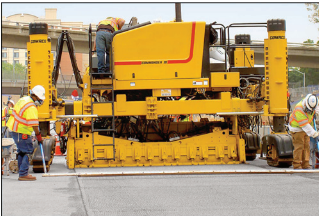
FIGURE 8 Placement and finishing fresh PPC surface with modified laydown machine and conventional tining rake. (Courtesy: Gomaco.)
