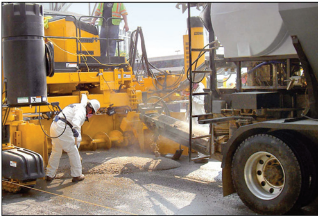
FIGURE 7 Metered mixing and placement of mixed polyester polymer concrete from mobile concrete batching plant. (Courtesy: Gomaco.)
