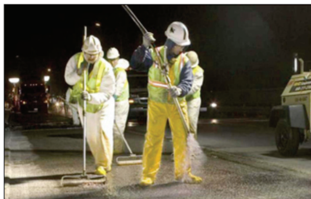
FIGURE 5 Priming deck with initiated high-molecular-weight methacrylate prior to placement of PPC. (Courtesy: American Civil Constructors.)
