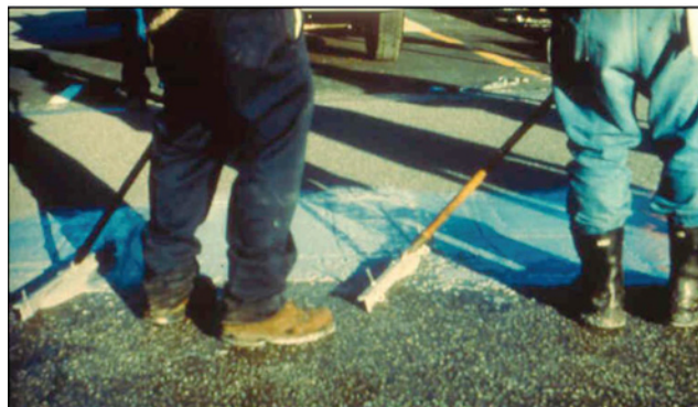
FIGURE 4 Using gauge rakes to control thickness of slurry overlay. (Courtesy: Virginia Center for Transportation Innovation and Research.)
