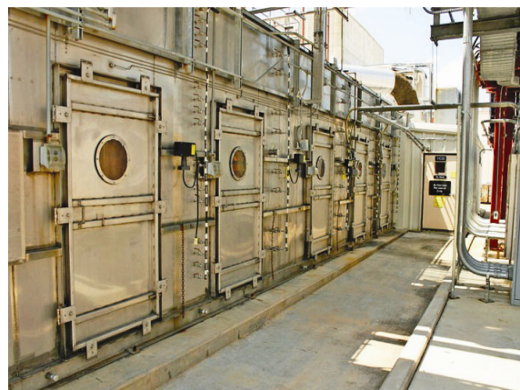
FIGURE 2-8 Vestibule on the side of an MDB HVAC unit. SOURCE: NRC, 2009b.
