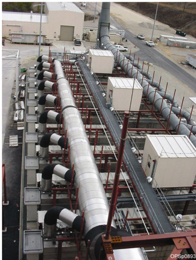
FIGURE 2-7 The nine activated carbon filter units for the MDB HVAC system. SOURCE: NRC, 2009b.
