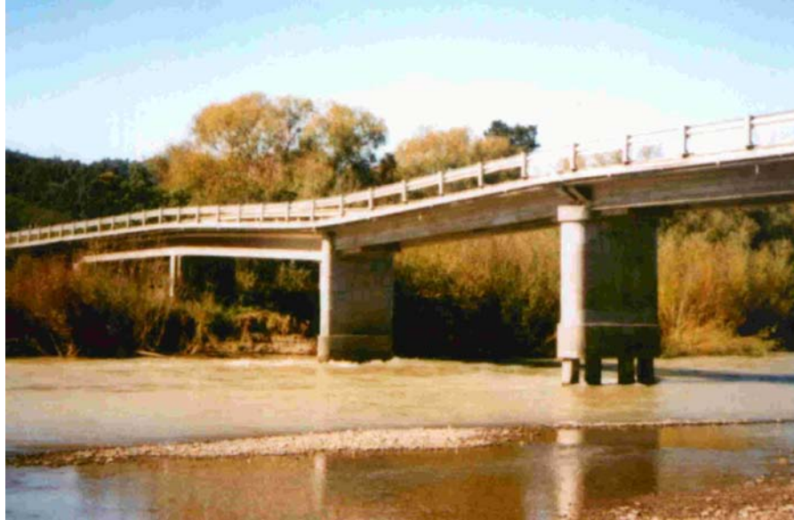
Figure 2-7 Bridge pier settled vertically owing to scour reduction of pier support
