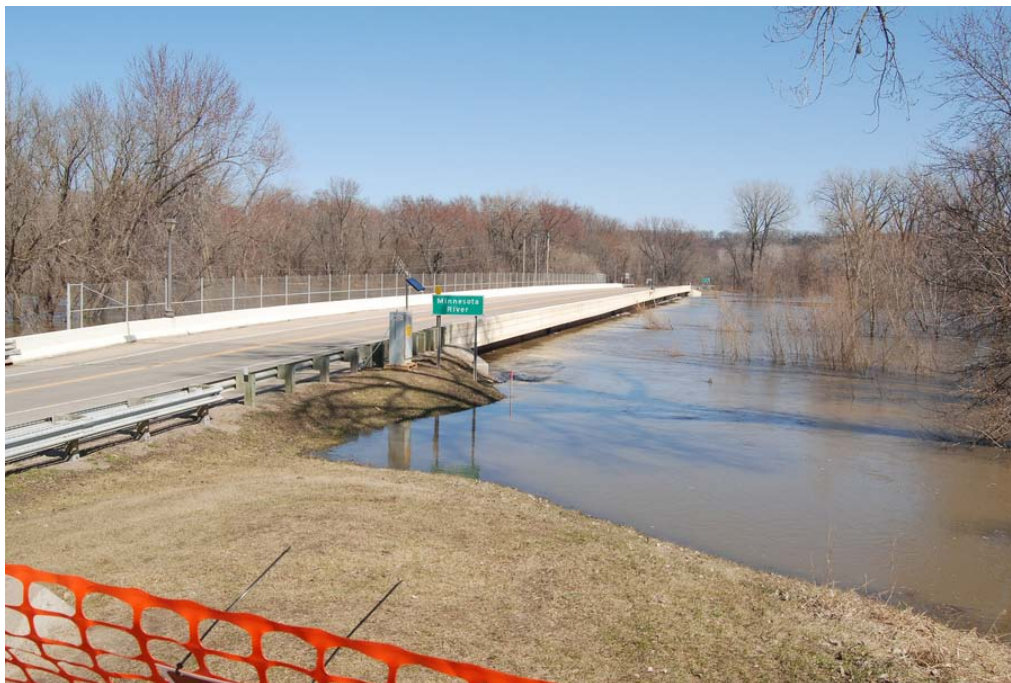
Figure 5-8 Bridge beams submerged by flood water
