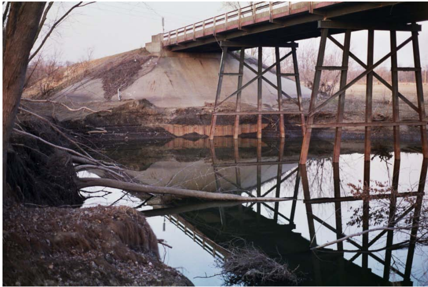
Figure 5-14 Pier scour and abutment/contraction scour on flood plain. Channel geometry and vegetation substantially affect the approach flow to the pier
