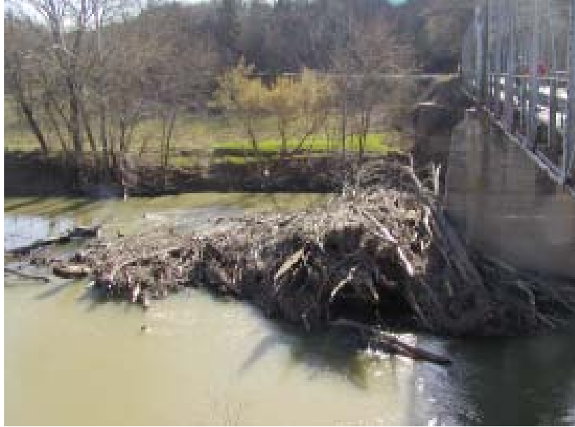
Figure 5-11 Woody debris accumulation at a single pier (Lagasse et al. 2010)
