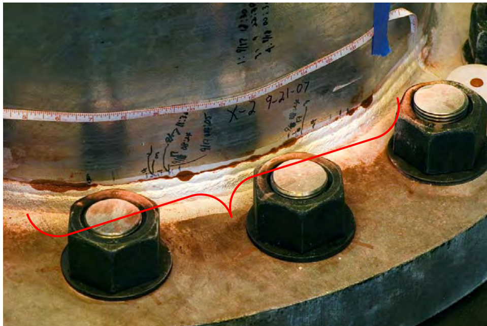
Figure 57 Fatigue cracking at pole-to-base plate fillet weld toe in high-level luminaire structure specimens
