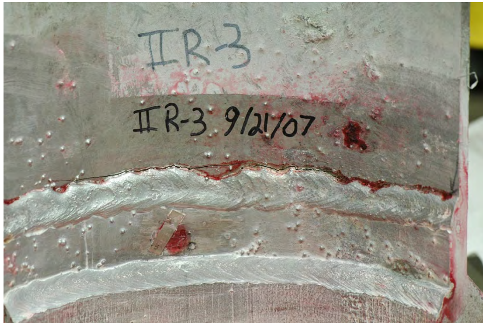
Figure 152 Quality of backing ring weld toe and fatigue cracking
