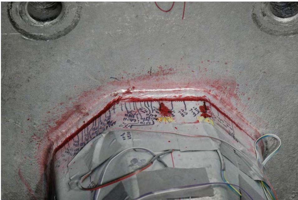
Figure 53 Fatigue cracking in arm of specimen VII-5, from the fillet weld toe on the tube in tube-to-transverse plate connection
