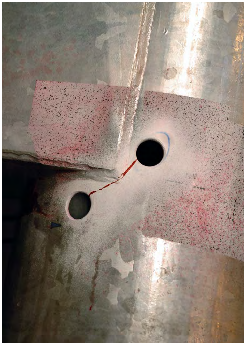
Figure 47 Fatigue cracking from gusset-to-pole fillet-weld in specimen IVB-1
