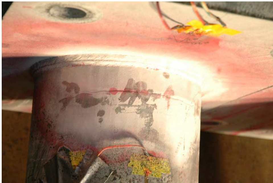
Figure 42 Fatigue cracking in arm from the toe of backing ring to tube weld (inside)
