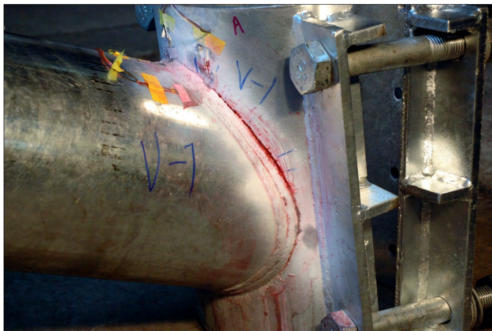
Figure 48 Fatigue cracking in specimen V from arm-to-clamp weld toe on the clamp
