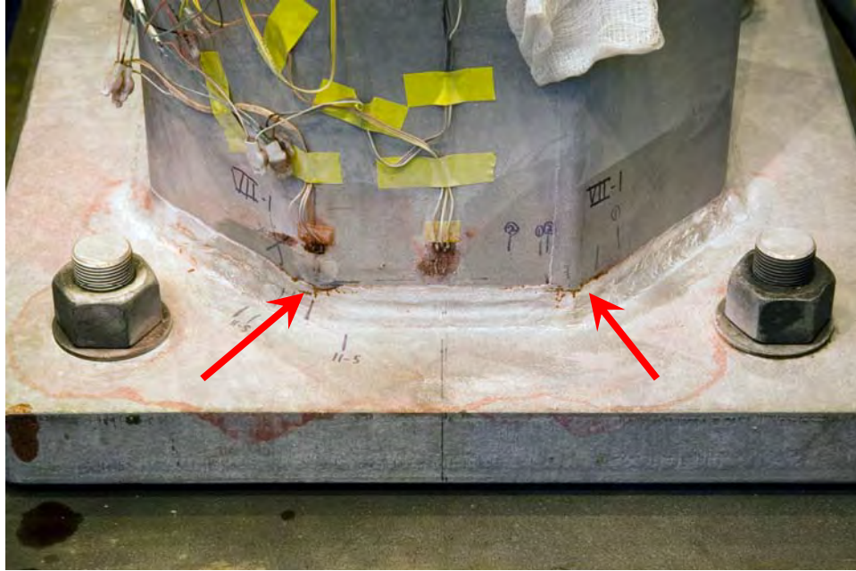
Figure 54 Fatigue cracking from toe of pole-to-transverse plate weld in pole of specimen Type VII
