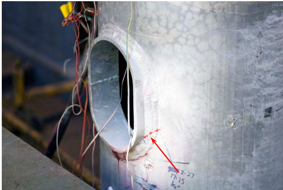
Figure 39 Fatigue crack from un-fused root of hand hole frame to pole weld
