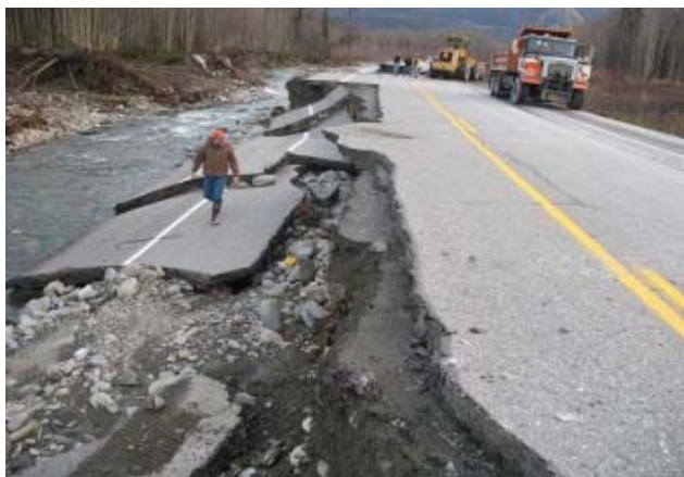
Damage on the Richardson Highway after unexpectedly high flood surges from the 2006 South Central Alaska storm.
