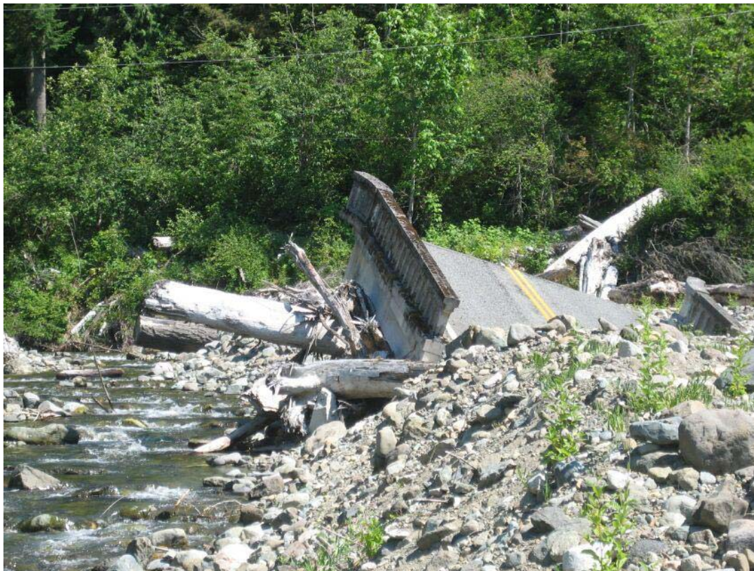
Scour and damage to structures, US-12 Davis Creek. (Photo courtesy of Washington State DOT.)
