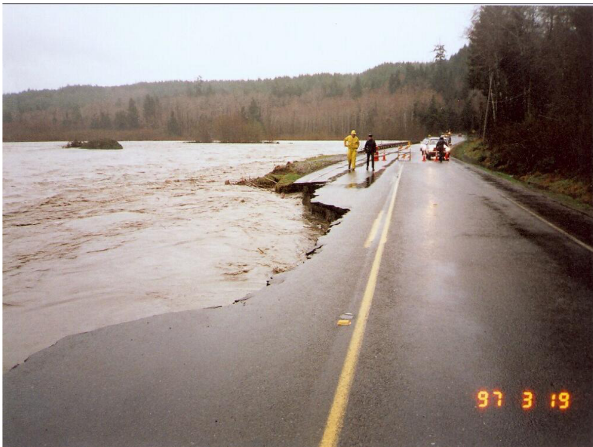
Changes in river dynamics: Hoh River flooding, channel migration, and avulsion. (Photo courtesy of Washington State DOT.)
