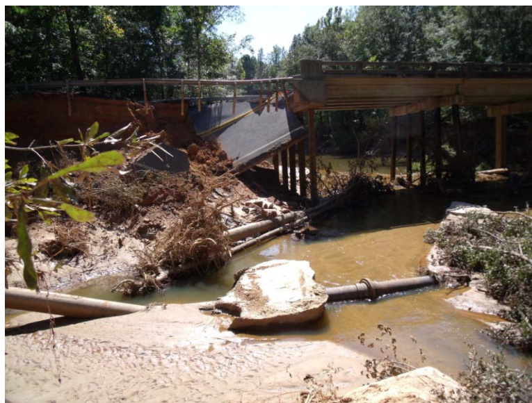
Figure 3-2. Failure of abutment fill in September 2009 Georgia flood accompanied by failure of approach roadway (Hong and Sturm 2010).
