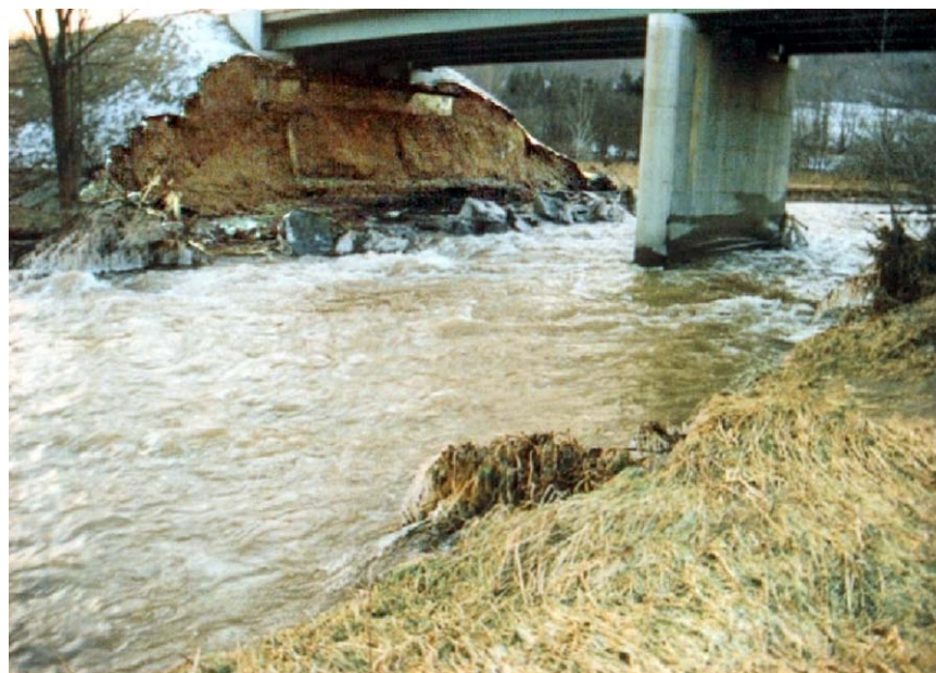
Figure 4-2. Field example of Scour Condition A.
