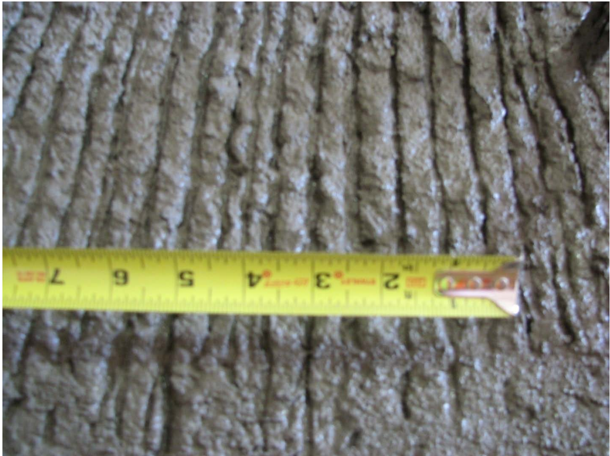
Figure 5.3.12: Intentionally roughened surface, by means of raking, of top web of precast beam used for the construction of Concept 2 laboratory bridge specimen
