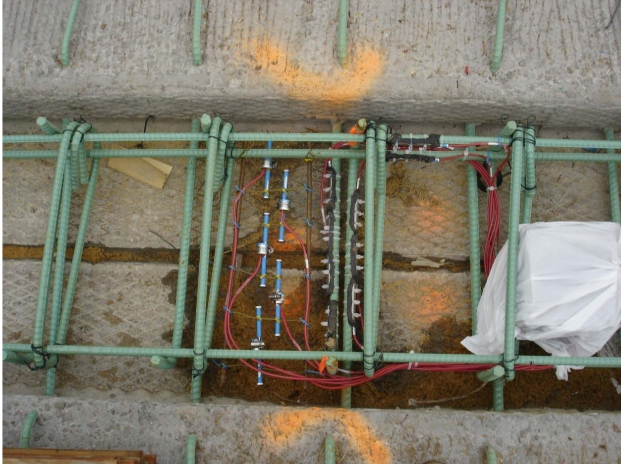
Figure 3.2.5: Lower level of concrete embedment and spot-weldable VW gages utilized in observation of reflective cracking in the Center City Bridge
