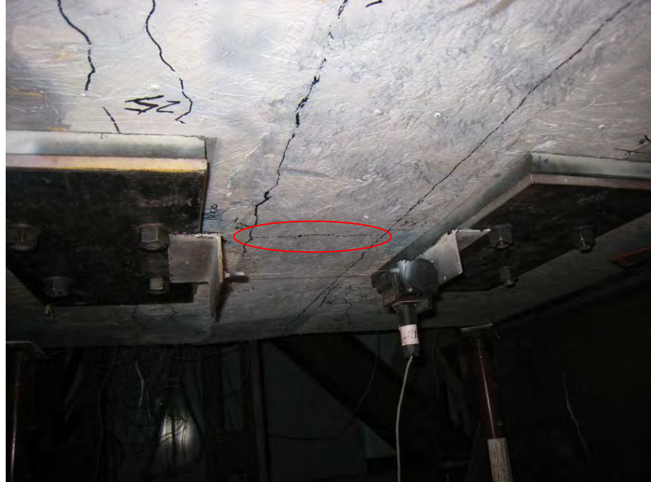
Figure 12.1.20: Transverse crack in FF-7 test (circled in red)
