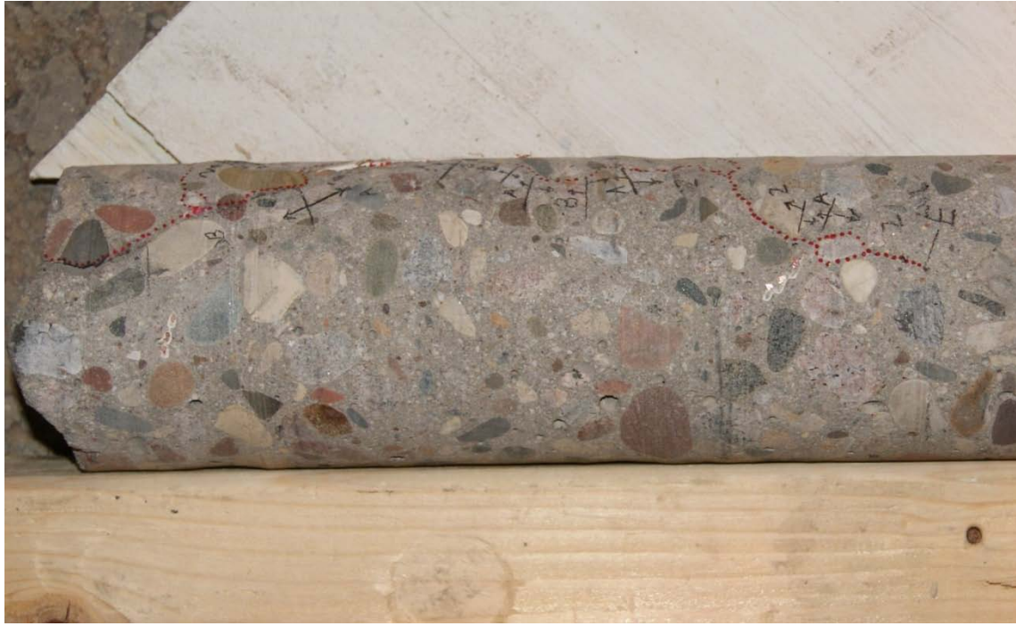
Figure G3: Crack widths marked on core specimen in pencil
