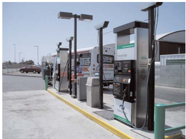
FIGURE 5 Oakland International Airport CNG fueling station.
