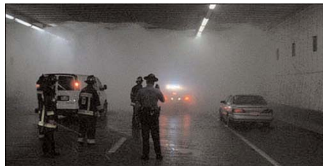
FIGURE 37 Accidental activation of the sprinkler fire suppression system in Boston CANA (Central Artery North Area Tunnel) for 45 min on May 15, 2005, at 2 p.m. (54).
