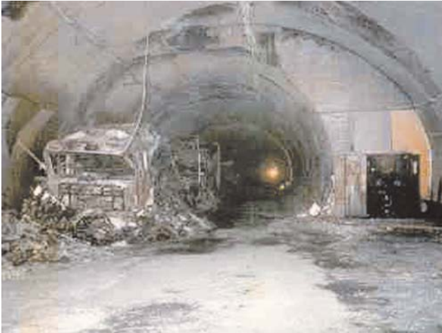
FIGURE 3 Mont Blanc Tunnel after fire.
