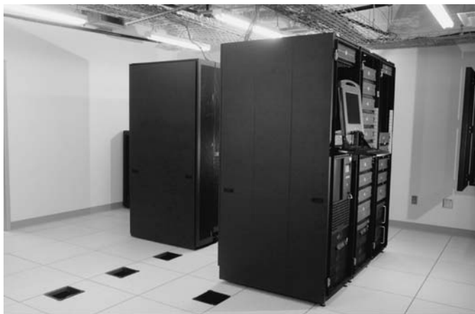
Figure 4.1. Environmentally controlled and secured VTTI data center.
