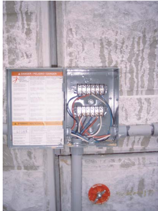
8. Typical junction box
