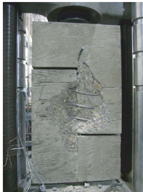
(b) Distortion of the interface steel reinforcement of specimen P1035-3A following large slip and cover spalling
